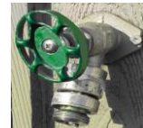
Hose bib with vacuum breaker installed
